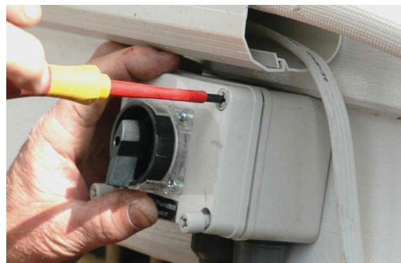
Figure 78: Install lockable isolating switch (C)
