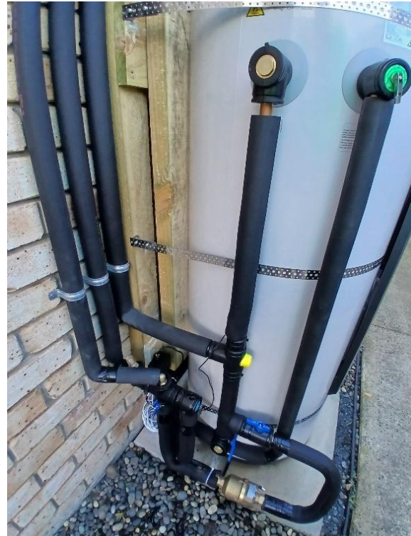
Figure 59: Seismic restraint for a hot water cylinder
