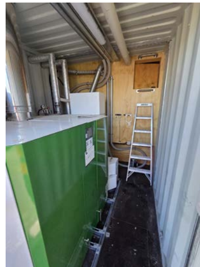
Energy Box Internal
