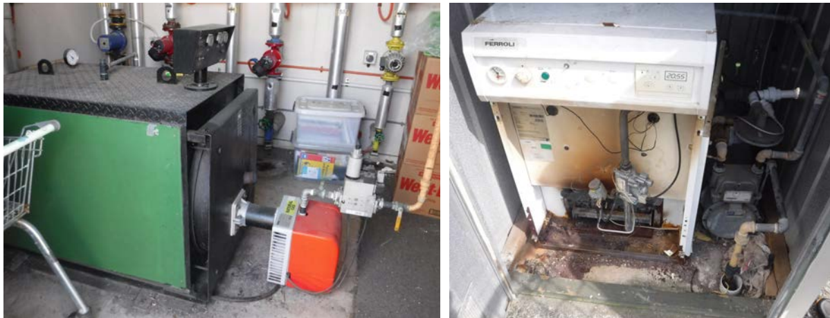
Figure 2: Previous Gas Boilers
