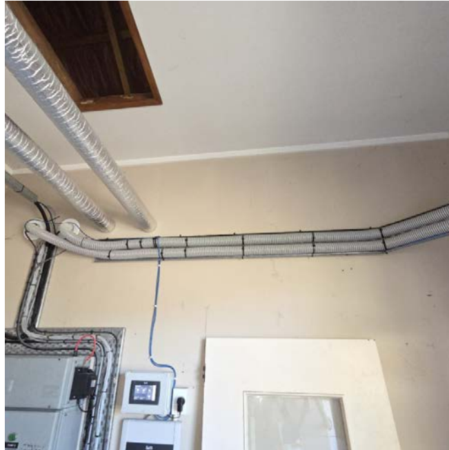
Flexi hose Supply Lines – Boiler Room
