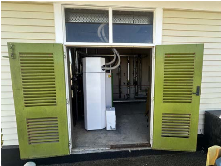
Existing Boiler House
