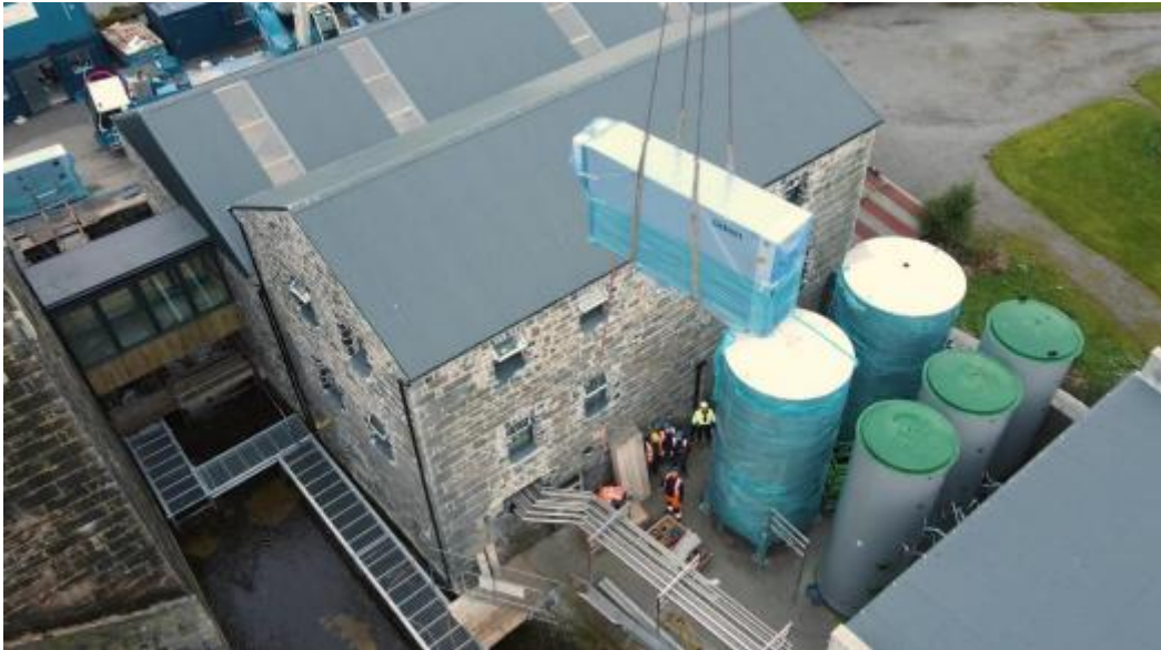
Figure 18. High-temperature heat pump being craned into services yard Source: Marren & Smyth (2026), p. 1; see footnote 28.
