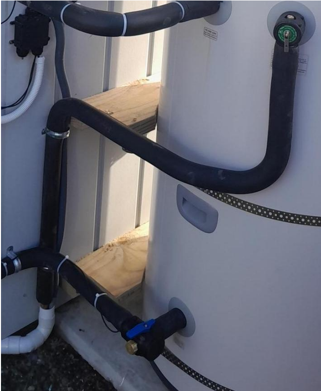
Figure 51: Temperature and pressure relief valve and discharge pipe
