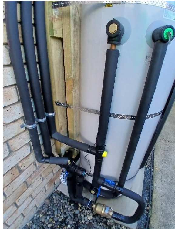
Figure 59: Seismic restraint for a hot water cylinder
