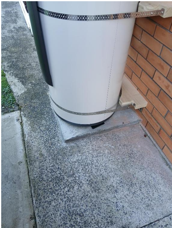
Figure 58: Seismic restraint for a hot water cylinder
