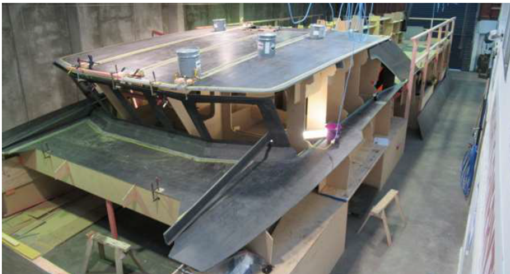
Photo: Progress with the construction of the carbon fibre deck at WEBB
