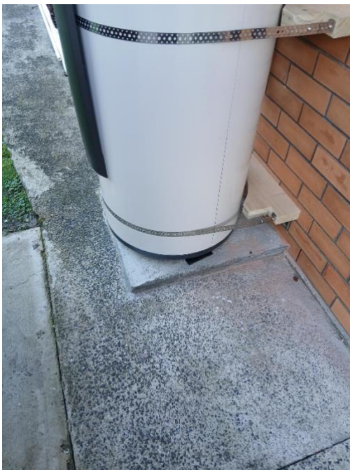
Figure 58: Seismic restraint for a hot water cylinder (A)
