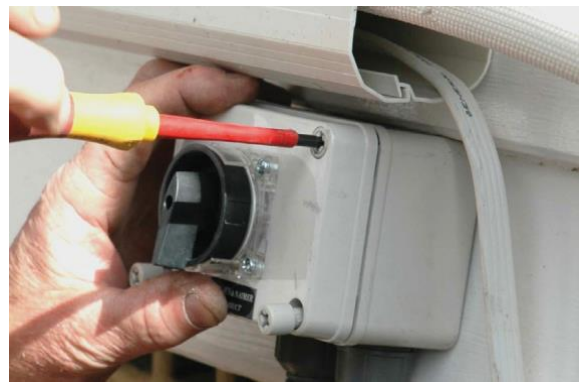
Figure 78: Install lockable isolating switch (C)
