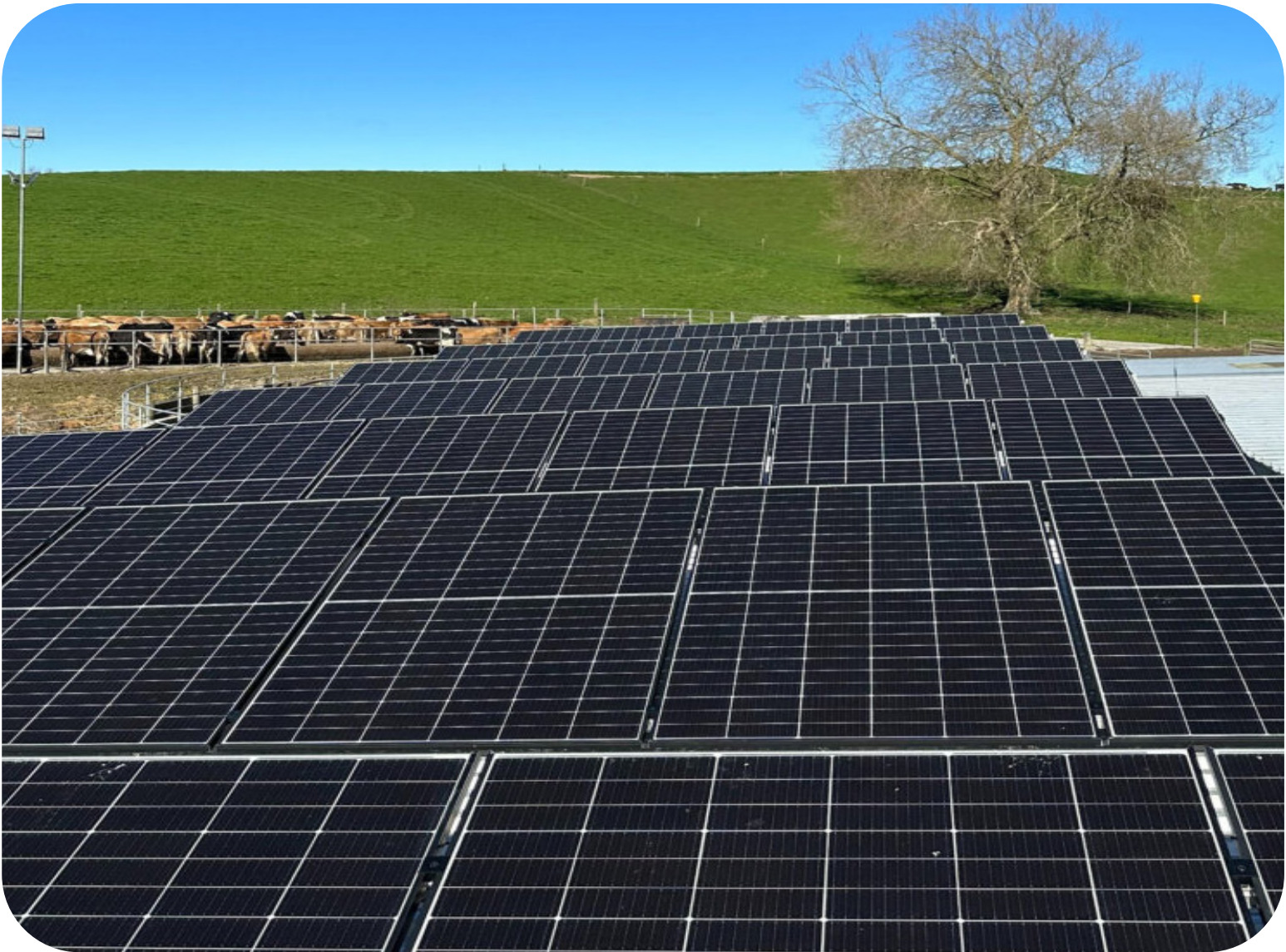
Commercial Solar Array Credit: Supreme Solar
