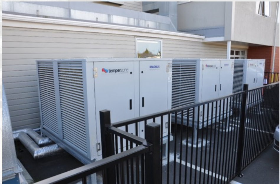
Decarbonised Energy Solutions' Magnus Variable Flow Water Heaters - Space Heating System, installed at George Manning Lifecare & Village
