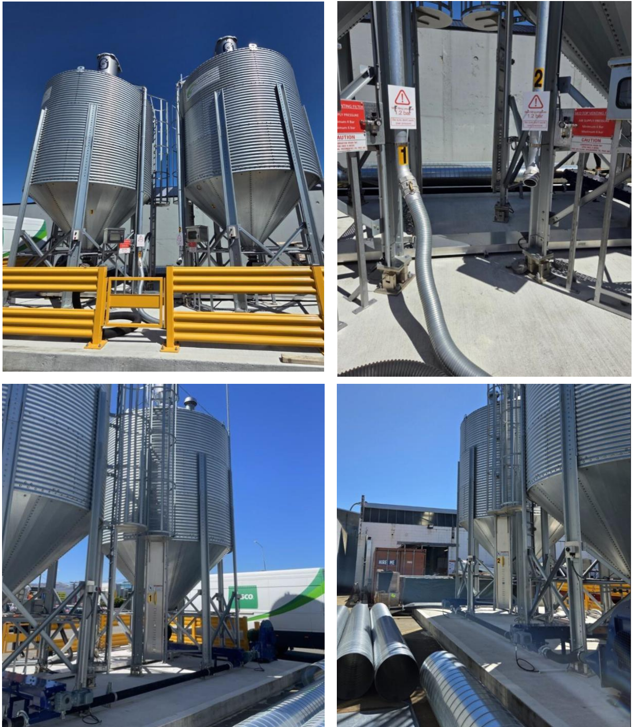
Figure 15: Silo System Photos
