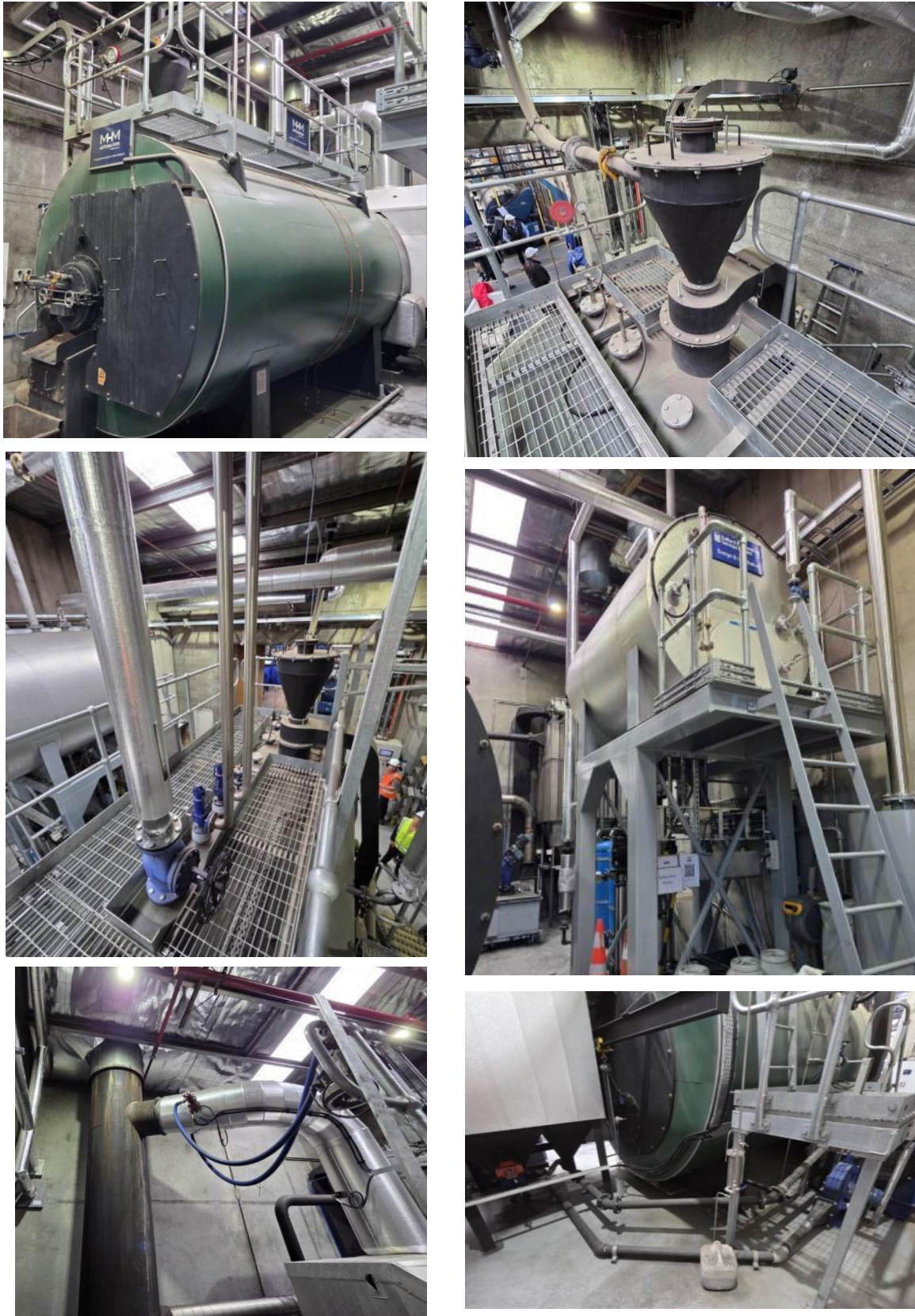
Figure 16: Boiler System Photos
