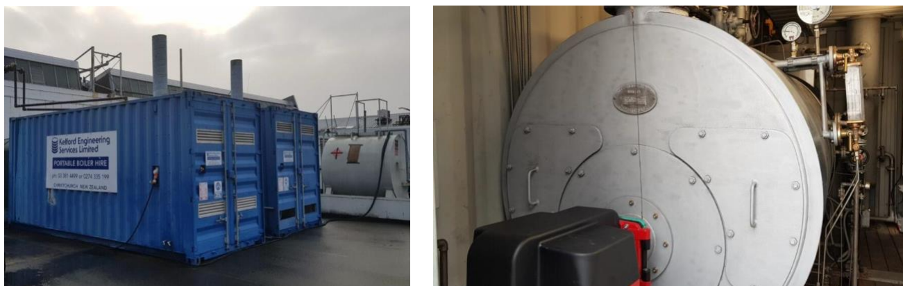
Figure 12: Temporary Diesel Boilers
