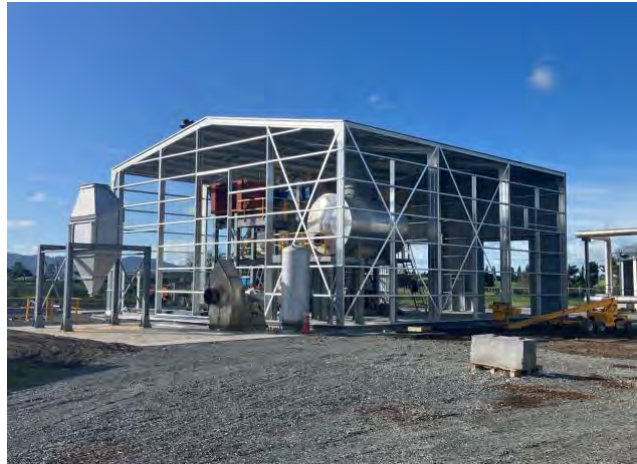
Boiler house and grit arrestor
