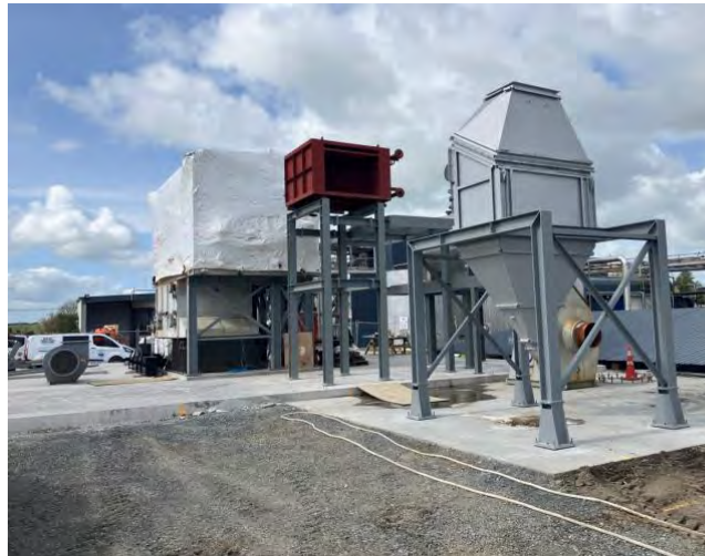
Boiler, economiser and grit arrestor
