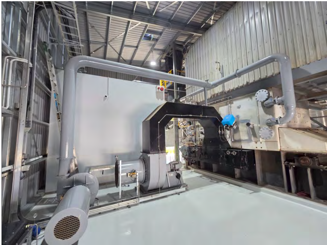
Forced draft fan for over fire and under fire air
