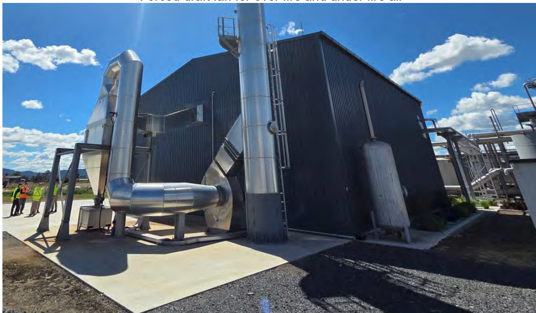
Particulate control is currently a grit arrestor with space to install further particulate control if required in the future. Photo shows forced draft fan and blow down tank.
