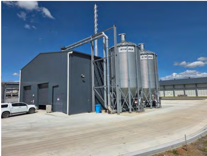
Pellet silos adjacent to boiler house
