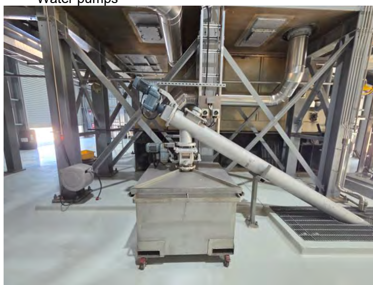
Bottom ash collection bin
