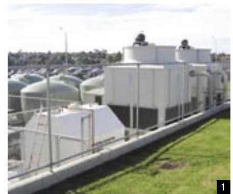
1 THE GREEN TANKS STORE STORMWATER. A DIESEL FUEL TANK IS IN FRONT OF TWO COOLING TOWERS THAT SERVE THE CHILLERS.
