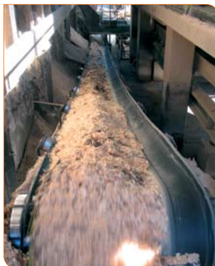
Mixed fuel for Boiler No. 2 is conveyed 10 metres up to the main feeder hopper.
