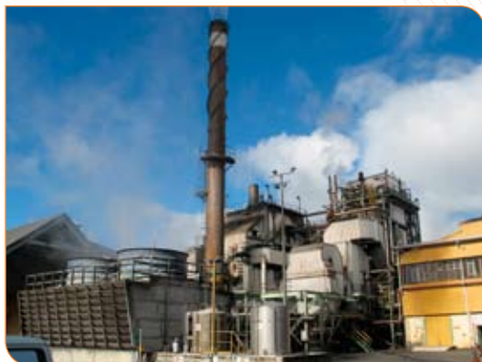
From left to right: Condenser unit, chimney, No. 2 boiler, No. 1 boiler, control room / turbine generator building.
