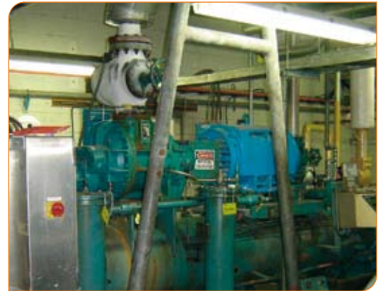
The compressor used to compress the ammonia gas during the chilling process.
