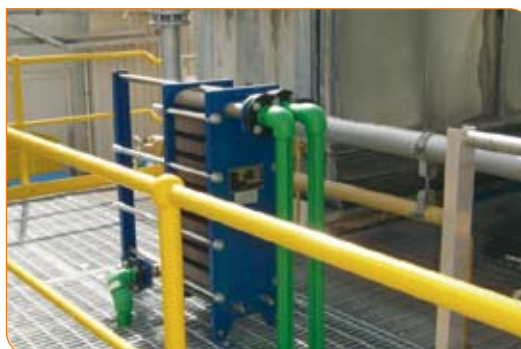
The plate heat exchanger - heat is absorbed by cold water from the town mains.
