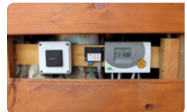
The monitoring equipment for the Eco Cabins is located behind a removable weatherboard, and can be incorporated into the education tour discussions.
