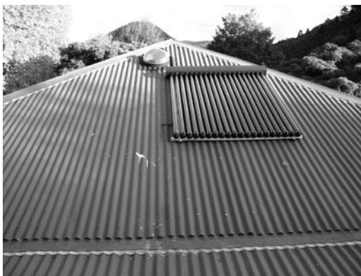
Figure 1: Evacuated tube solar collector panel installed on corrugated iron roof (photo by Emsol)
