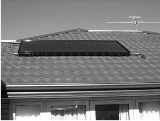
Figure 4: Flat-plate solar collector panel with pipe insulation weather protected (photo by Emsol)
