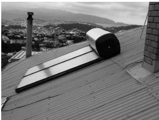
Figure 2: Flat-plate solar collector panel with hot water cylinder mounted on the roof (photo by Emsol)
