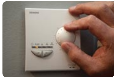
Upgraded room controllers provide efficient air conditioning control and give guests greater flexibility in setting their level.
