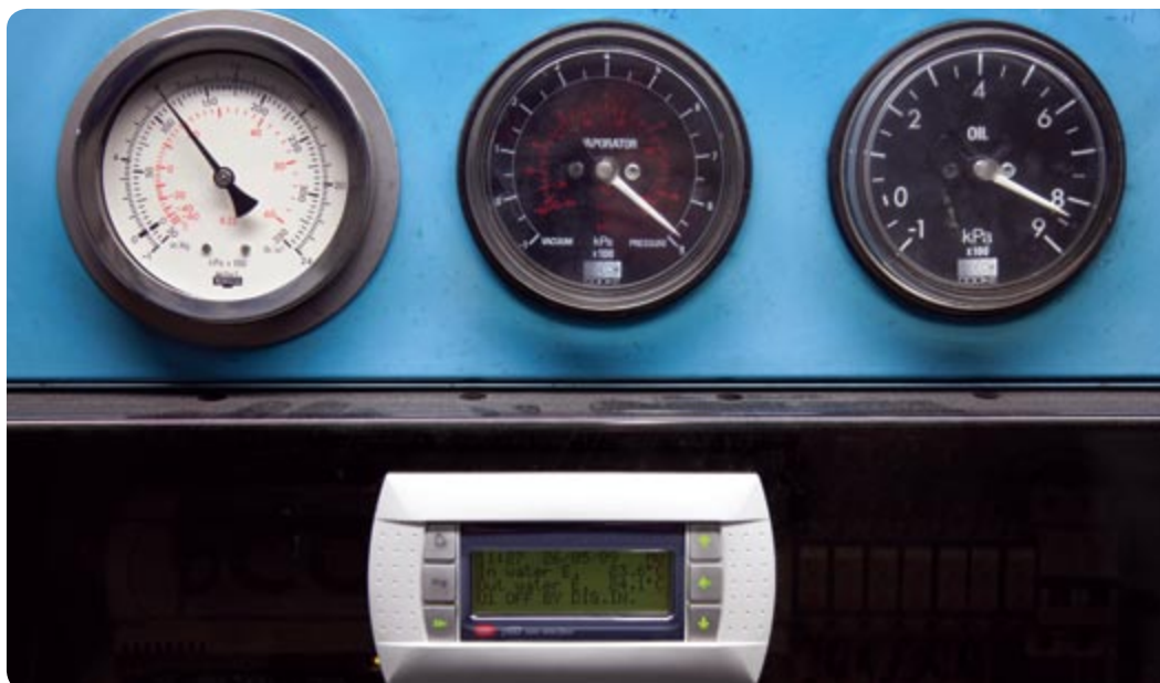
Original fit chiller controls are superseded by a retro fitted microprocessor control providing greater reliability and flexibility of operation.
