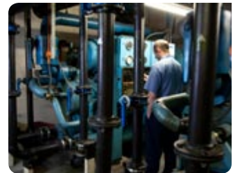
Adjustments are made to chiller parameters using upgraded technology controlling legacy plant.
