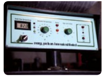
The original LPG boiler control provides feedback to the Building Management System.
