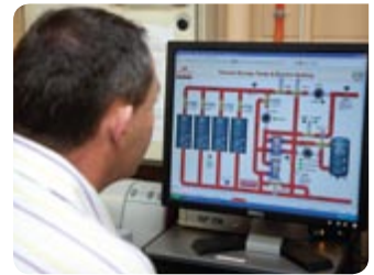
The new Building Management System computer integrates the new and old.
