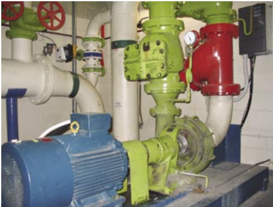
THE BLACK PANEL ON THE WALL IS A VARIABLE-SPEED DRIVE (VSD) , WHICH CONTROLS THE SPEED OF A GREEN CONDENSER PUMP AND BLUE MOTOR .
