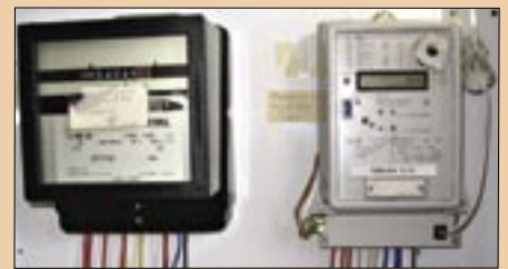
ELECTRICITY METERS, WHICH ASSIST IN MONITORING PEAK LOADS
