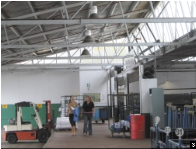
3 BEFORE, HIGH-BAY LIGHTS IN THE LOADING DOCK WERE LEFT ON UNTIL SOMEONE THOUGHT TO SWITCH THEM OFF. NOW, A DAYLIGHT SENSOR SWITCHES THEM OFF WHEN DAYLIGHT IS ADEQUATE.
