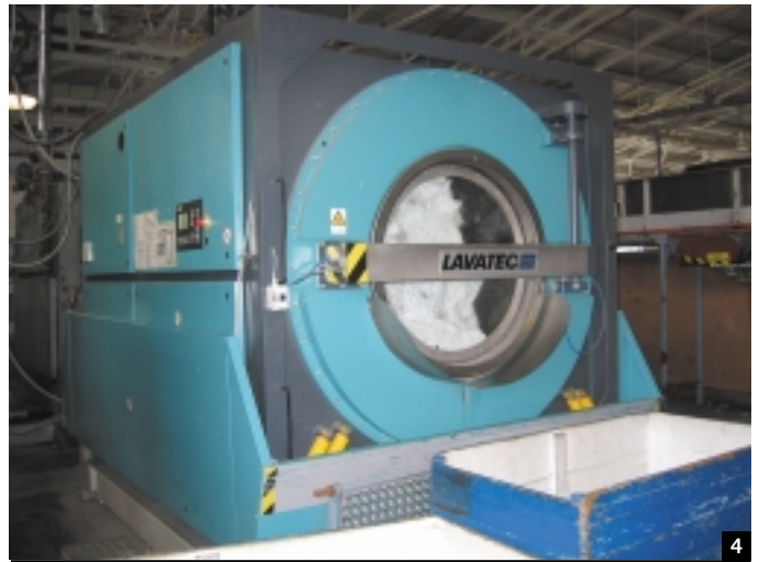
4 THE LAVATEC WASHER COMES WITH THE LATEST VARIABLE SPEED DRIVE USING A SINGLE MOTOR DRIVE . THE WASHERS ARE MORE EFFICIENT THAN OLDER TYPES THAT REQUIRED UP TO FOUR MOTORS.
