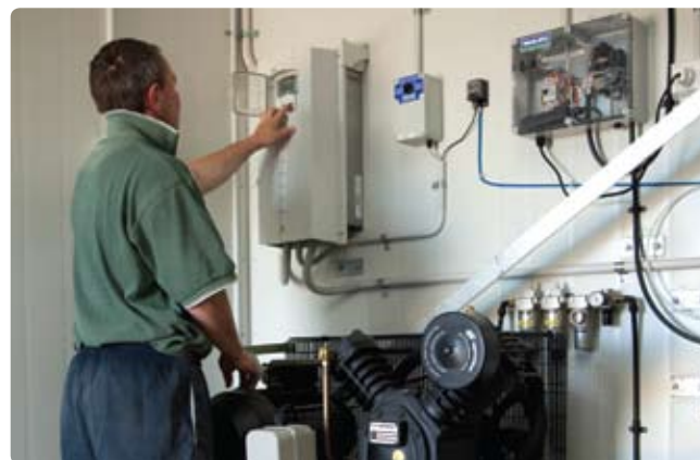
Monitoring of energy usage on the variable speed vacuum pump controller.
