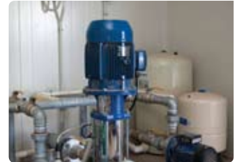
Variable speed water pumping reduces energy use and water hammer, and extends pump life.
