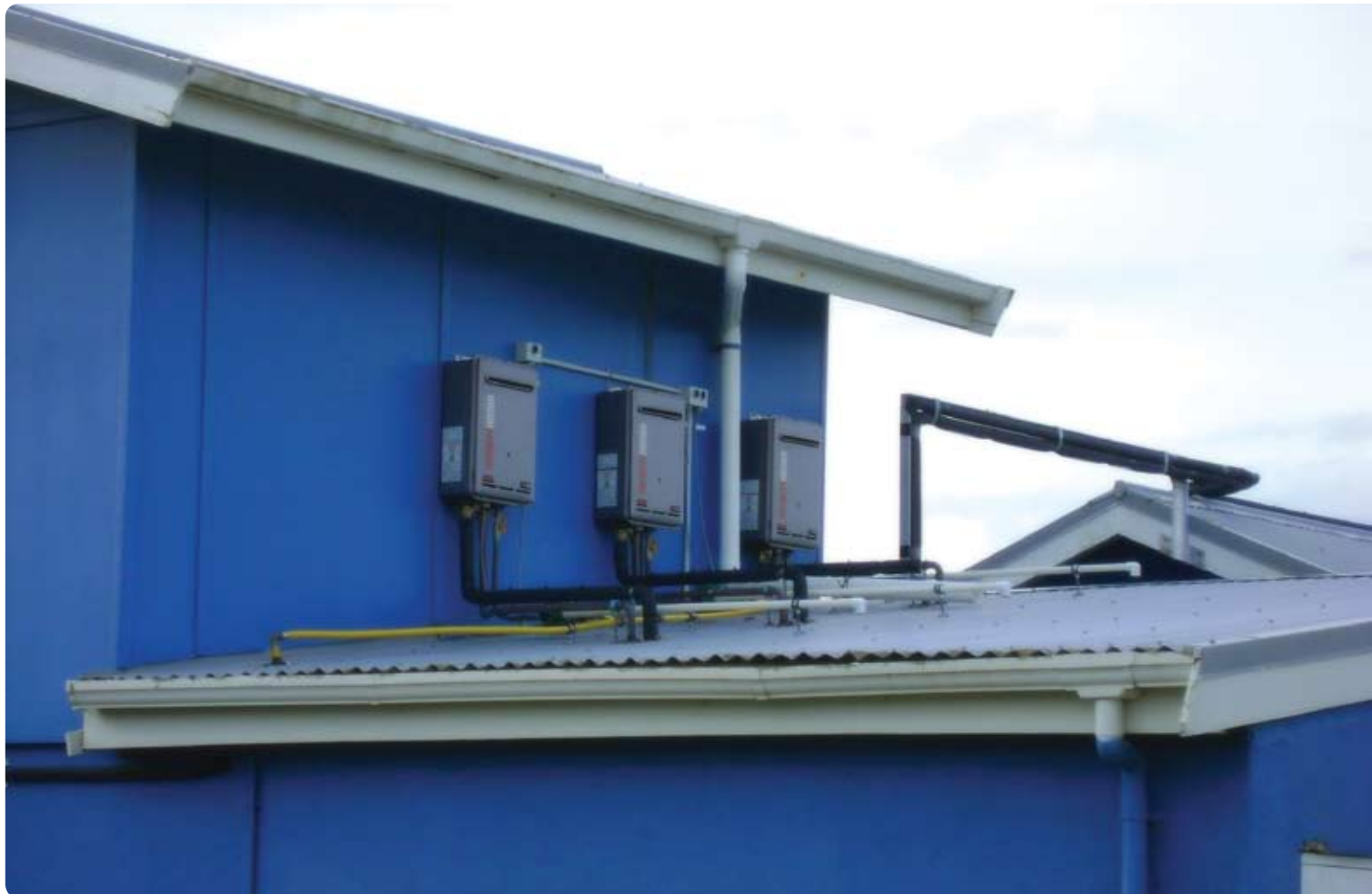
The three Rheem 26 gas heating units top-up the heat in the three cylinders below when needed.
