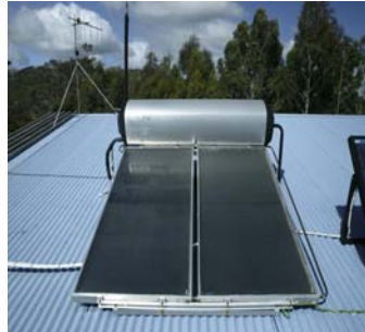
4 m 2 flat plate collector with horizontal tank
