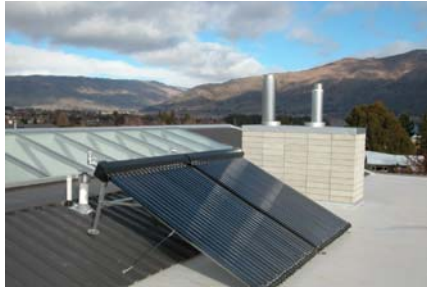
Evacuated Tube System
