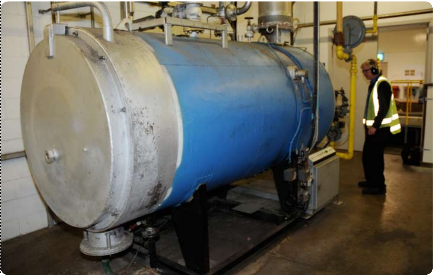
The old steam boiler at Pernod Ricard
