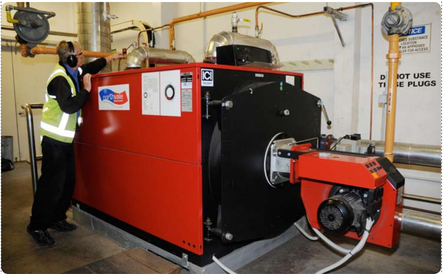
Pernod Ricard's new hot water boiler
