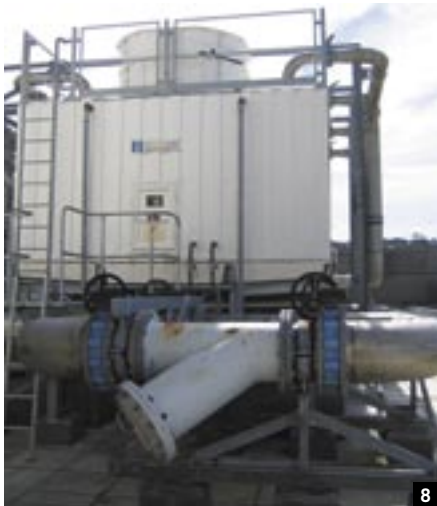
8 ROOFTOP COOLING TOWER. THE TEAM IS PLANNING A SMART ENERGY TECHNIQUE WHERE WATER COLDER THAN THE USUAL 25-26°C IS SPRAYED THROUGH THE OUTGOING AIR. FOR EACH DEGREE COLDER, 3% LESS COOLING TOWER ENERGY IS NEEDED.
