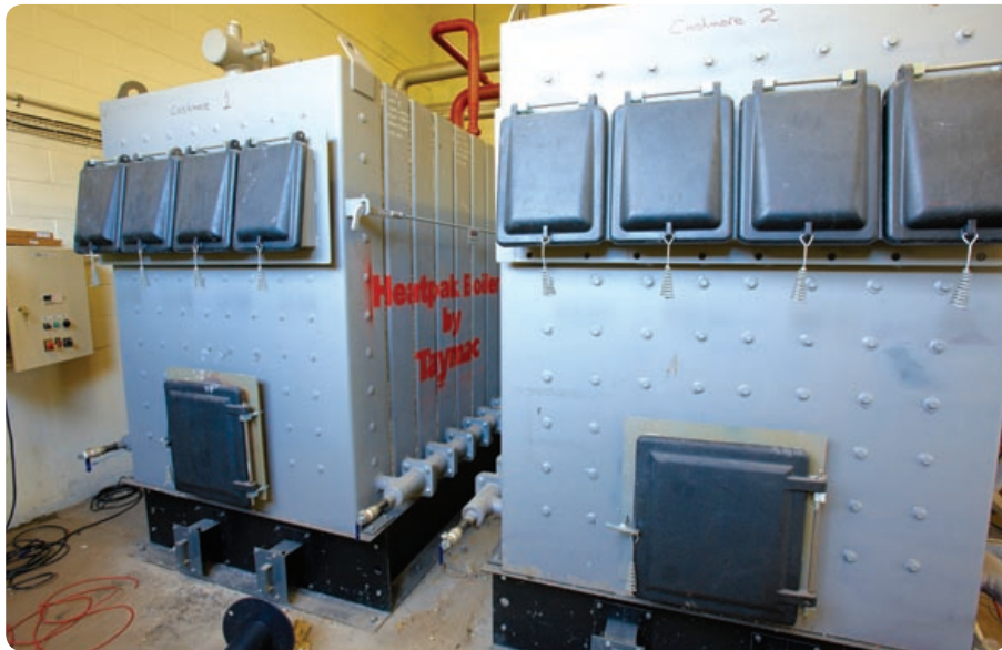
Two 640 kW wood-fired boilers.
