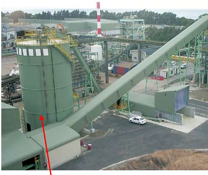
Silo (800m 3 , 10m diameter and 18m high)
